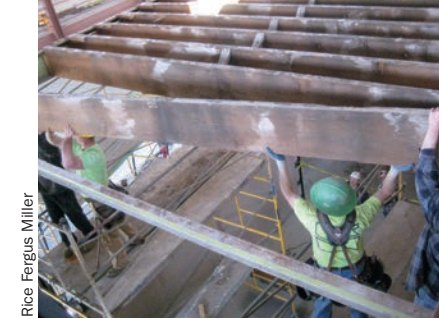
Workers remove the upper floor beams to create the open forum space. The 1948 vintage Douglas fir is repurposed through the space.
